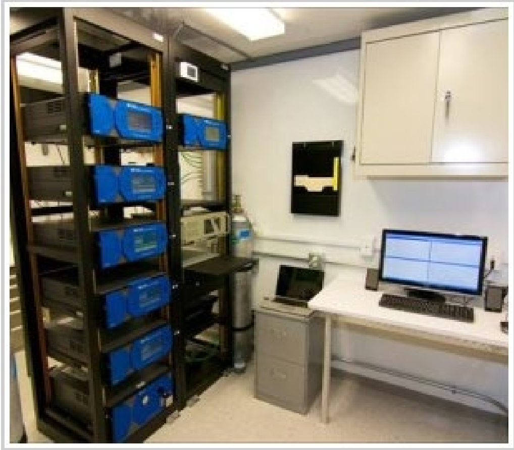
Source: Air Monitoring Equipment Shelters | Shelter One
