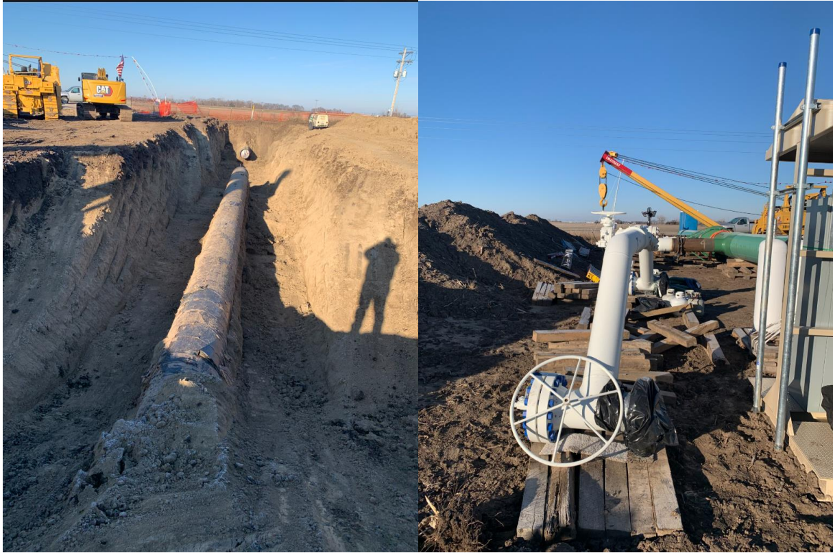
Figure 1: Pipeline and Safety Shut Off Installation on the DGRS farm outside Glenville, Nebraska
